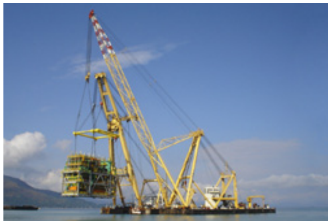
Dockwise MV Transshelf engaged in a 'float-over' for the OFON 2 project, offshore Nigeria, for Technip/Total
