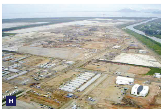
G Aerial view reclamation site of steel plant H Aerial view construction works in progress for steel plant
