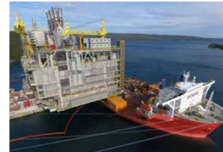
BULL ARM, NEWFOUNDLAND The load-out of the 42,000mt Hebron Utilities Process Module from the Blue Marlin
