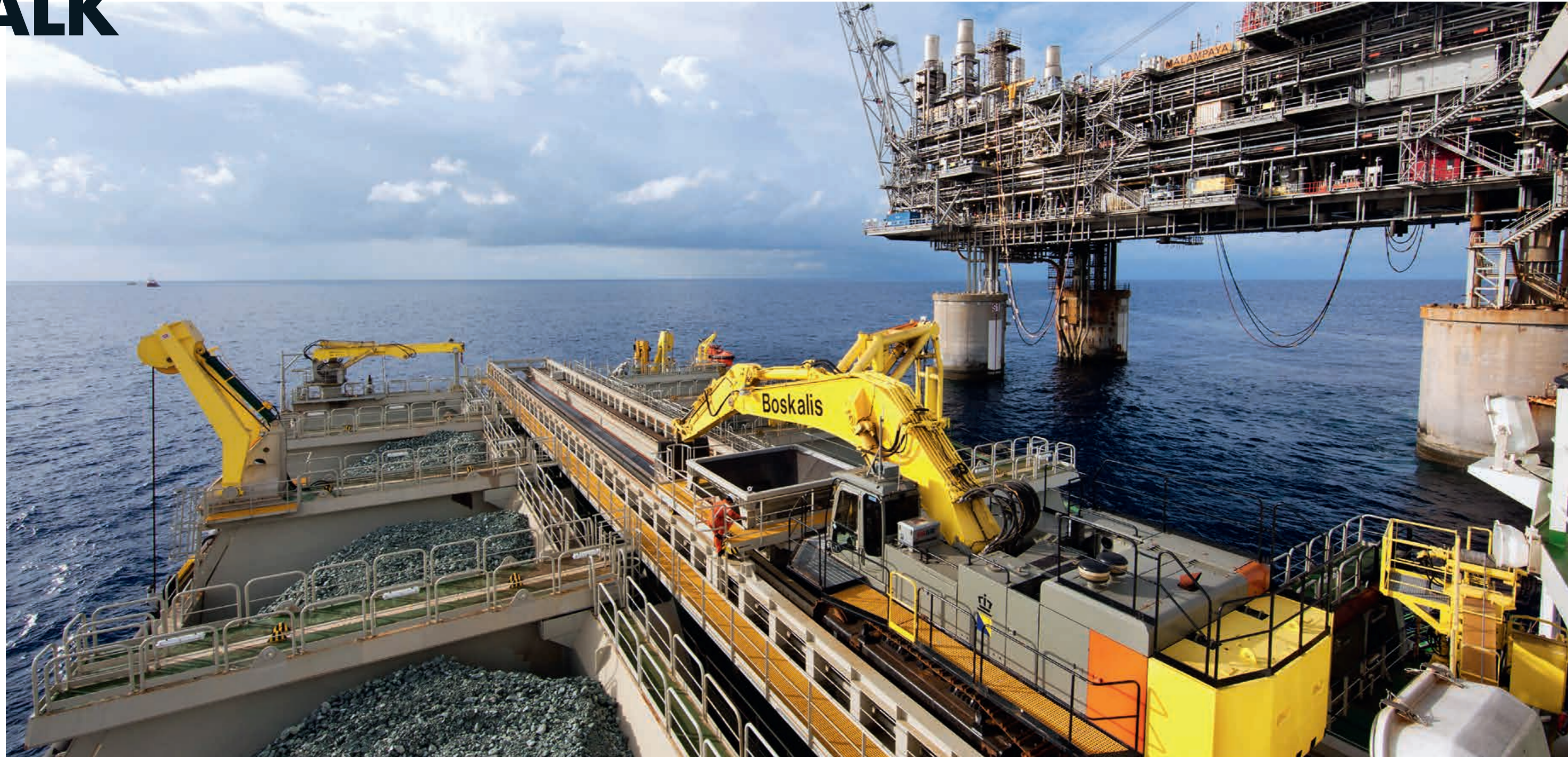
MALAMPAYA FIELD, PHILIPPINES Seabed preparation works with the Ndeavor for the installation of the Depletion Compression Platform in Malampaya gas field.
