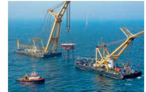
NORTH SEA Taktif 4 and 7 taking part in the preparation and removal of the QAB platforms from the Dutch Continental Shelf.
