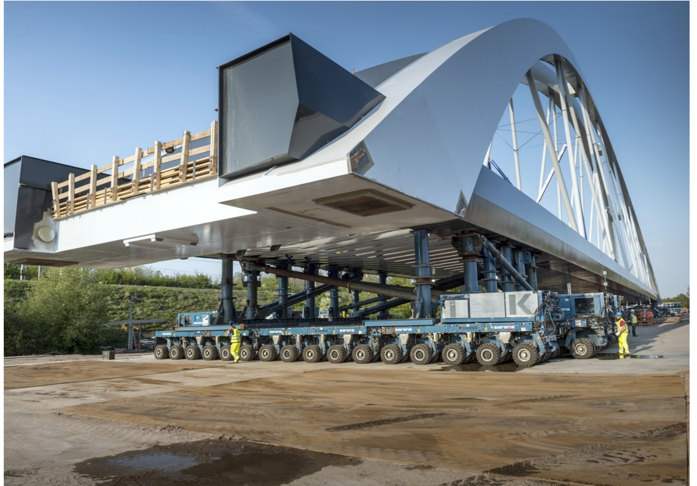
SAAONE, THE NETHERLANDS Soil improvement specifically designed for the installation of a 8,400 ton weighing rail road bridge to prevent soil failure and the safety risk that the structure would slide from the installation vehicle.
