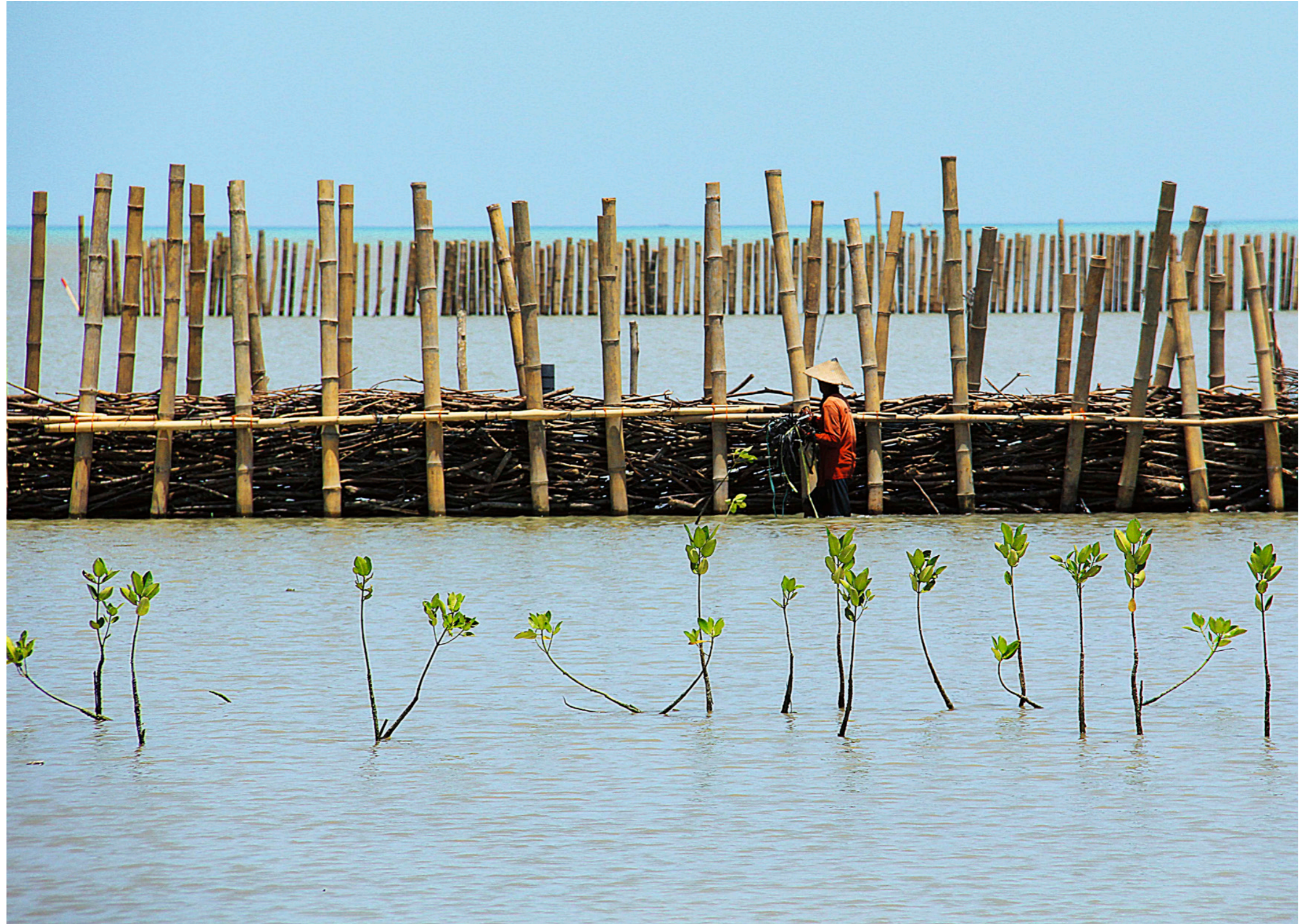
MANGROVE RESTORATION, INDONESIA Construction of permeable dams made from bamboo poles and brushwood to facilitate the large-scale restoration of mangrove forests. The aim of this project in Central Java is to develop a stable, sustainable mangrove coastline that can adapt to rising sea levels while enabling local economic development. These dams dampen the waves and take the energy out of the water, while the sediment can still filter through, accumulate and settle behind them. Mangroves can then grow behind the dams and not be washed away by the waves.
