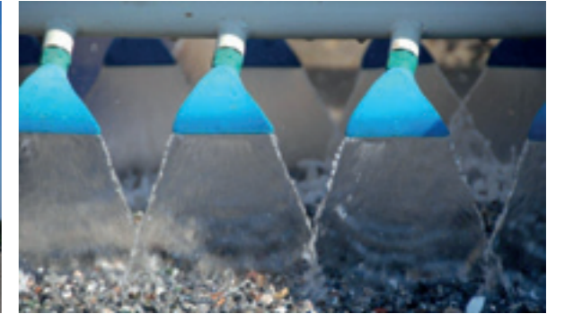
top middle TORONTO, ONTARIO, CANADA Construction of the Mobile Soil Washing Plant, for the Toronto Soil Recycling Demonstration Project.
