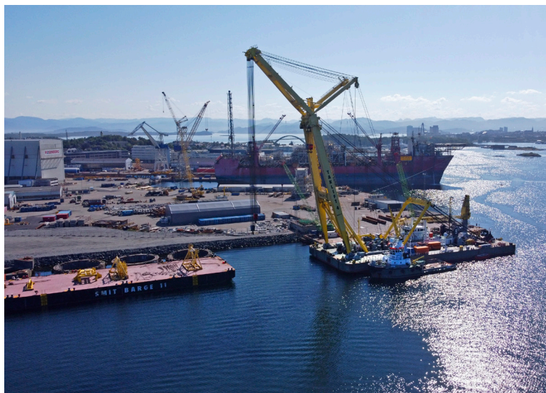
A Marine Spread: Taklift 4 in Fly-Jib configuration, tug Sapphire and Smitbarge 11 B Lifting of upper Gantry
